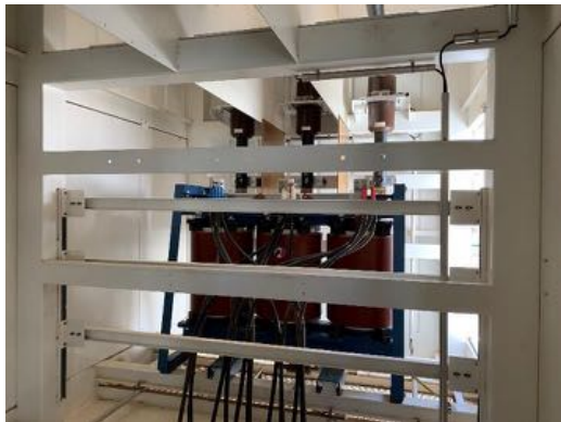
Picture: UPS Auxiliary Transformer
